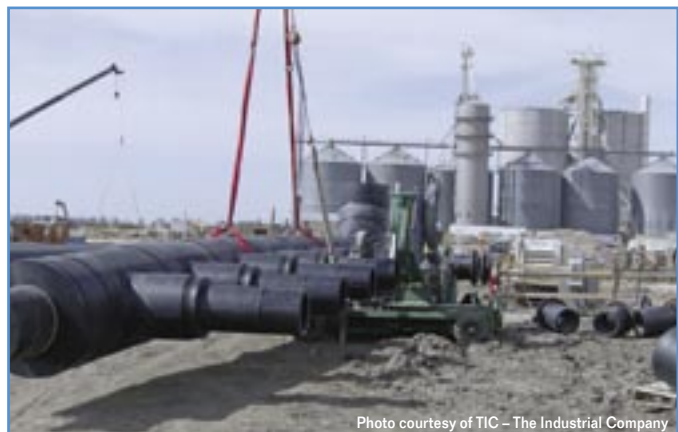
ISCO custom fabricates HDPE structures at their fabrication plants or on the jobsite, as shown above with this 42" fabricated header for chilled water application at an ethanol power plant.
