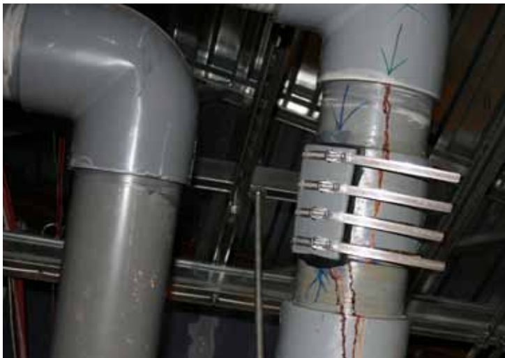
An example of the leaking CPVC pipe that needed to be replaced. This shows leaks around the joints.
