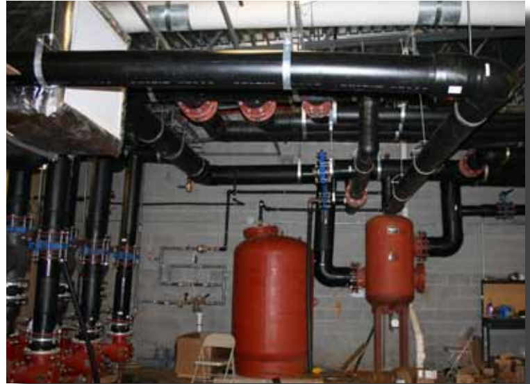
An example of some of the prefabricated pipe sections provided by ISCO Industries to help speed up the installation process and minimize the amount of welds or fusions that needed to occur onsite.
