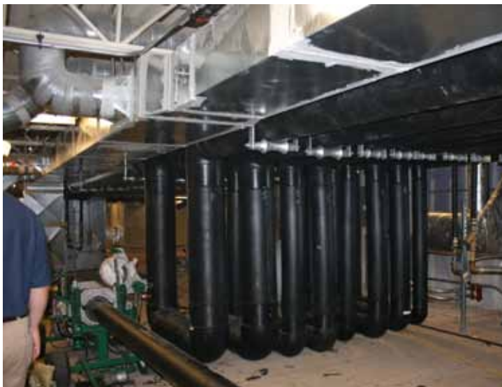
A closer look at the complex nature of some of the sections of the piping system. This shows HDPE pipe already in place along with a McElroy fusion machine being used to fuse more pipe.
