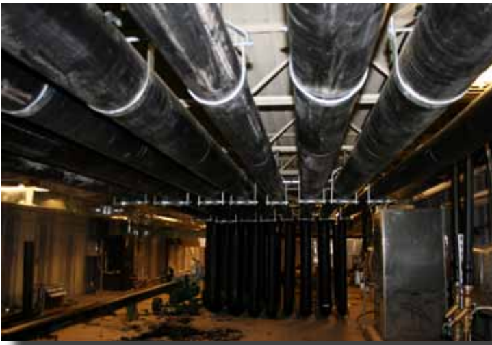
The piping system is complex and runs through various sections of the school. This section or zone of the geothermal piping system now made of HDPE is located above the common kitchen and serving areas for the high school and middle school's cafeterias.
