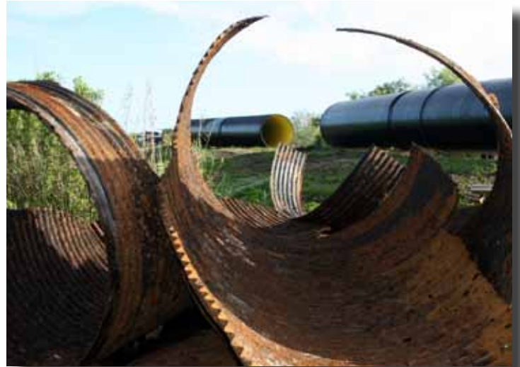
A view of the excavated deteriorated corrugated metal pipes with the new profile wall pipe liner in the background.
