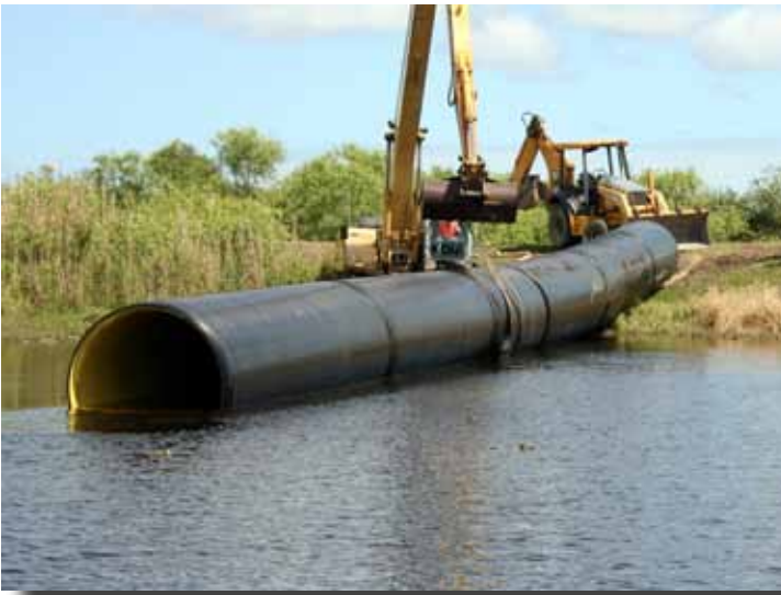
The electrofused PPT pipe was placed in the water to be submerged under water and pushed into the old pipe.
