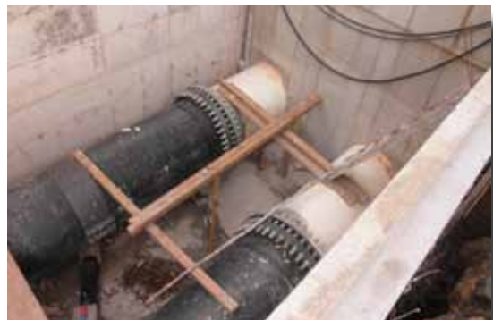
Pipe connected inside a tank.
