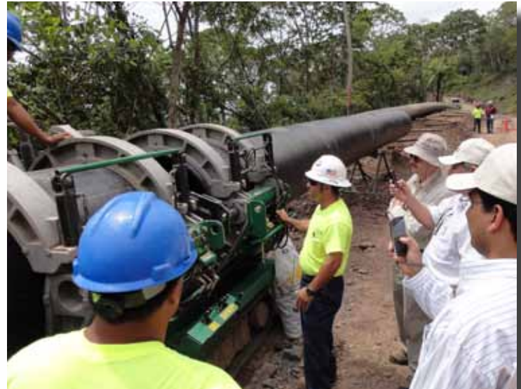
The HDPE pipe is fused onsite while visitors observe the fusion process.
