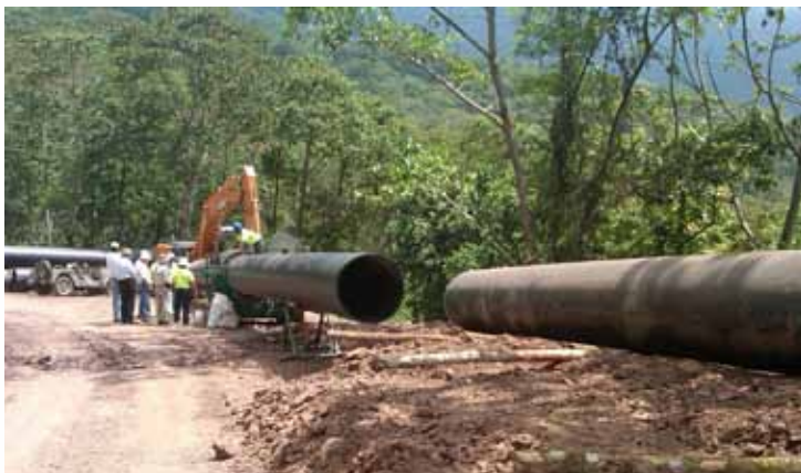
After the HDPE pipe was fused it was installed underground and eventually connected to a tank. The flow of the water will power a turbine, generating power.
