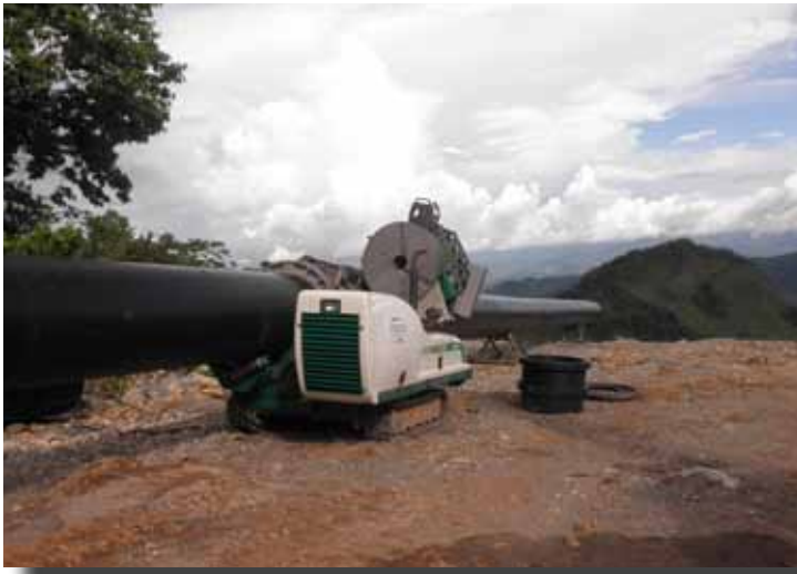
A view of the HDPE pipe along the hilly landscape characteristic of this part of Guatemala.
